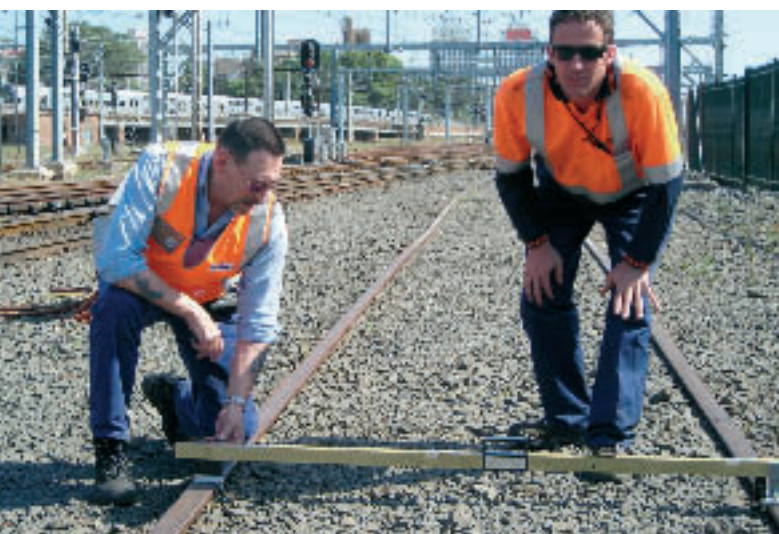
POOR MAINTENANCE: "It's all been very frustrating," says rail union member and track maintenance employee Tom Jones, pointing to the deterioration of safety and the widespread use of unskilled casual labour to increase profits.
