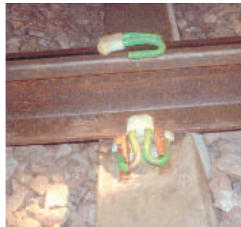
TWISTED SLEEPER: This sleeper is deformed and several clips are not secure
