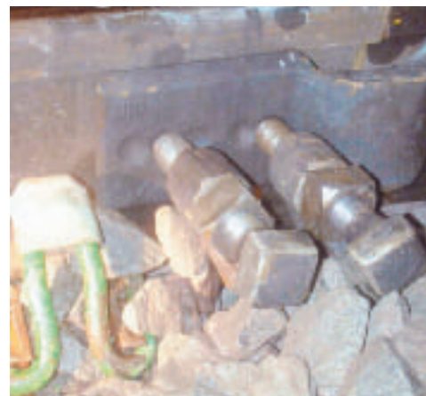
LOOSE BOLTS: Two rails that need welding are held by a clamp resting on ballast and the bolts are not tight
