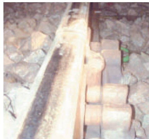
MISALIGNED TRACK: Two pieces of track don't line up
