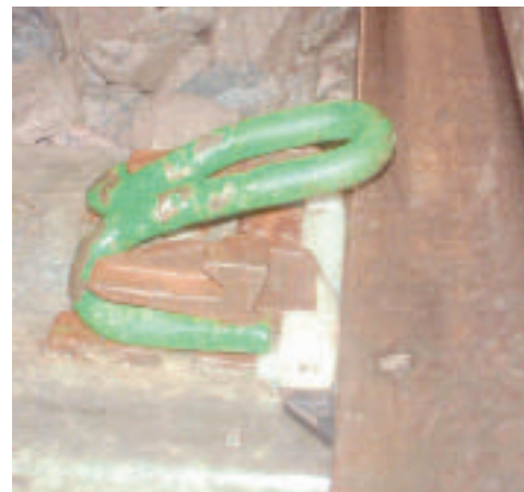
LOOSE CLIP: Loose clip not holding the rail
