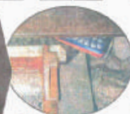
DANGER: Phone fits in gap between a sleeper and rail
