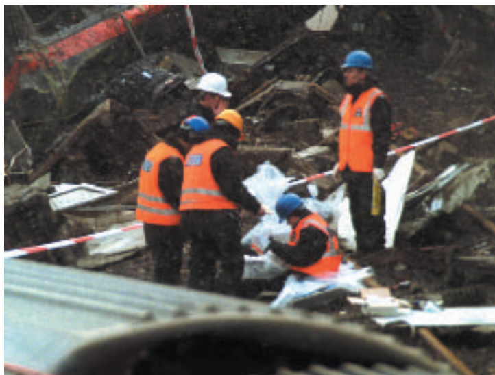
WRECK: Police forensic and accident investigators sift through the wreckage of the train Selby rail crash, Great Heck near Selby, Yorkshire. Photo: Mark Pinder
